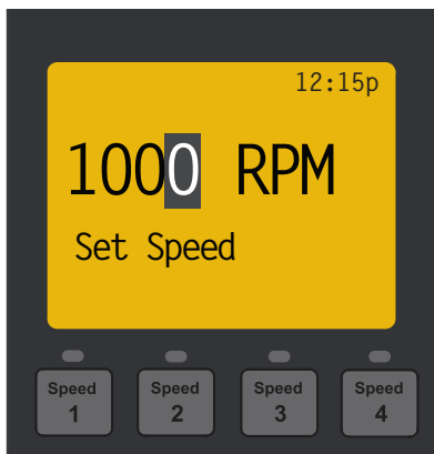
Setting the Anti Freeze Pump Speed
