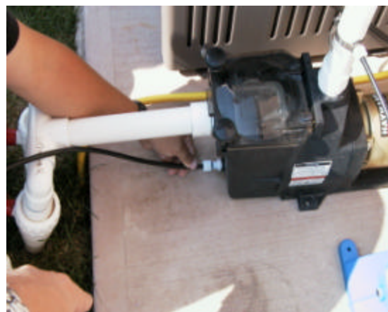
Retrofit into the Strainer Basket
