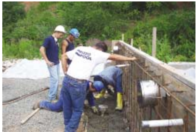
Photo 1: Setting main drain in a fictitious pool wall. Rizzo personnel showing Denis Beaupré (in blue hardhat, kneeling) how to set main drain.
