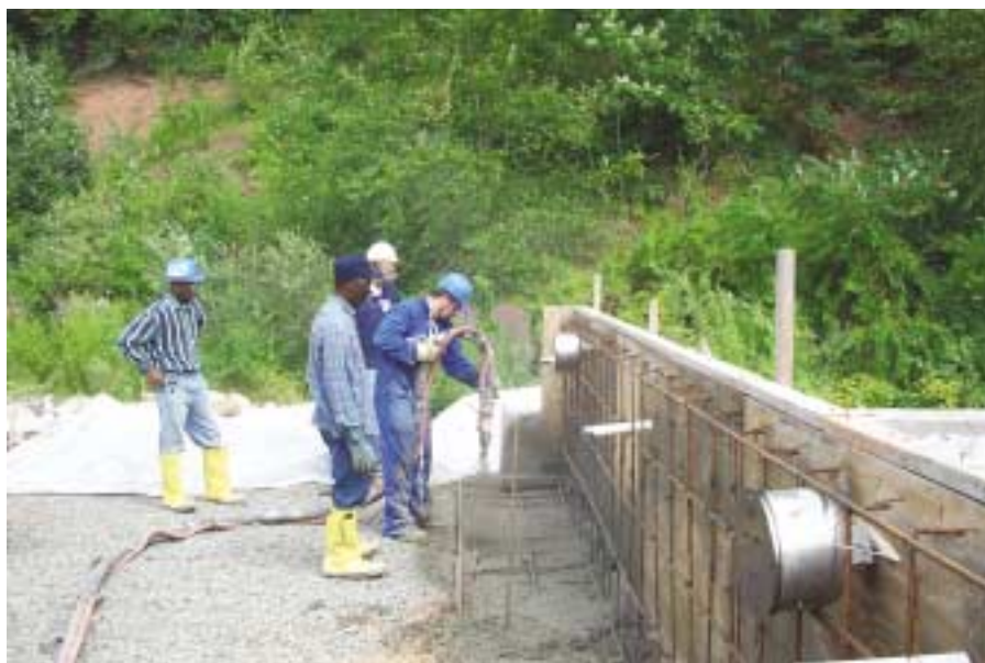
Photo 3: Professor Denis Beaupré instructs three Rizzo employees shooting simulated pool floor and wall, the proper procedure for shooting floor.
