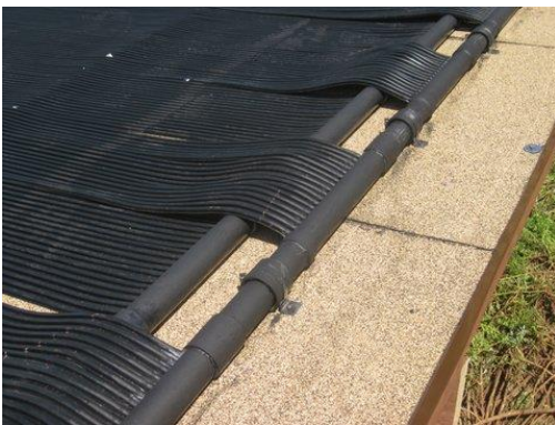
Staggered headers with pvc pipe on a rack installation
