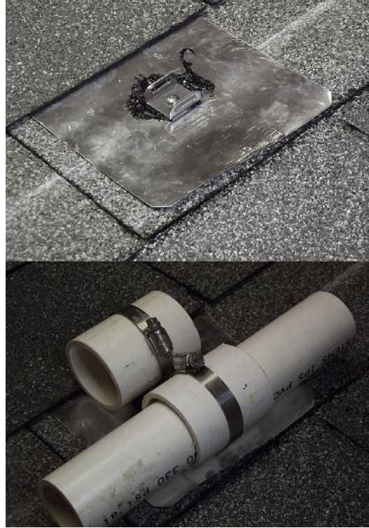
slip collars supporting a plumbing run on a shingle Roof – 2 strap brackets, one screw
