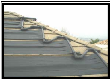
Connecting the headers of a staggered system.
